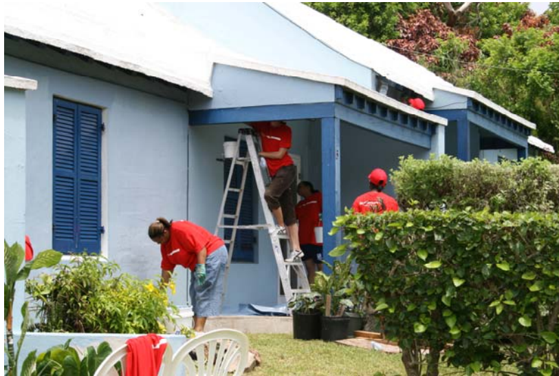
Bank staff painting the homes at the Bermuda Housing Trust's Elizabeth Hills complex
